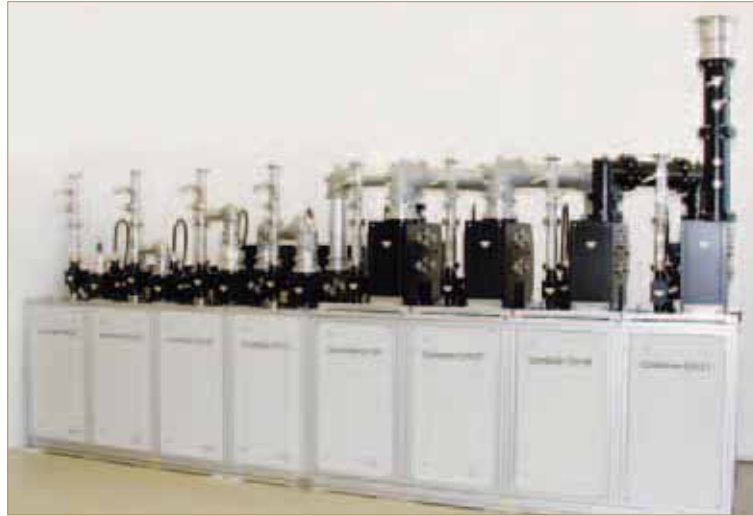
BN 57 54 02 Rennes, France UHF combiner for 8 x 5.6 kW DVB with integrated mask filters and monitoring couplers
